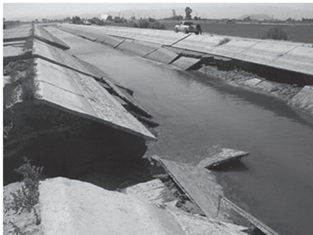
Damage to transport infrastructure
